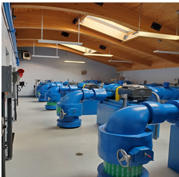
Puetz Booster Station
